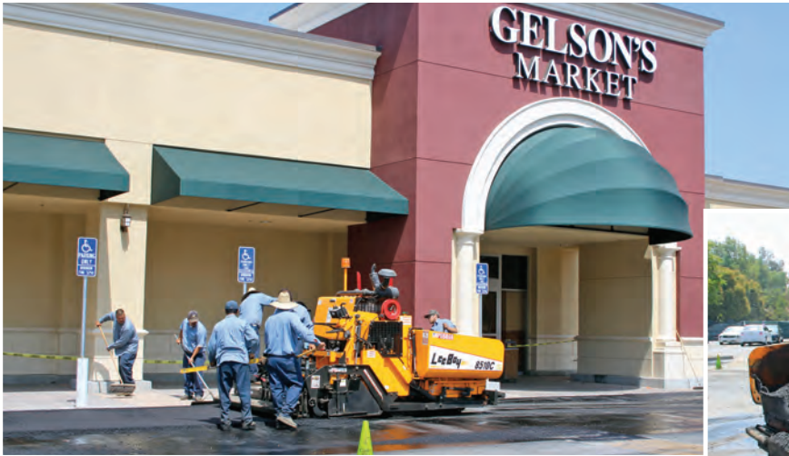
Above: Competitive Asphalt Coatings, Inc. uses their brand new LeeBoy 8510C on a patch and pave project at Gelson's Market in Sherman Oaks.
