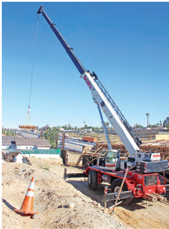
Right: One of (2) Link-Belt RTC 8090 Series II cranes purchased especially for the Interstate 805/ Palomar Street bridge replacement and addition of on and off ramps as well as new retaining wall construction in Chula Vista for Granite Construction.
